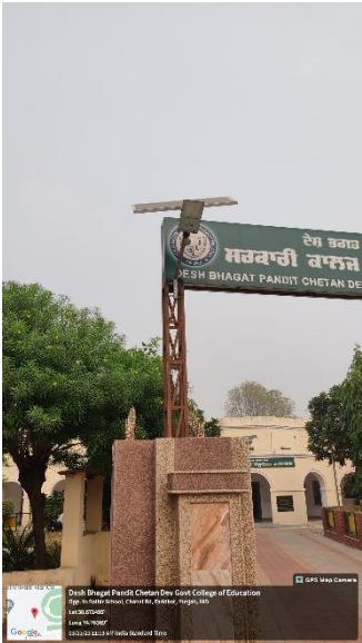
33. Solar Street Lights
